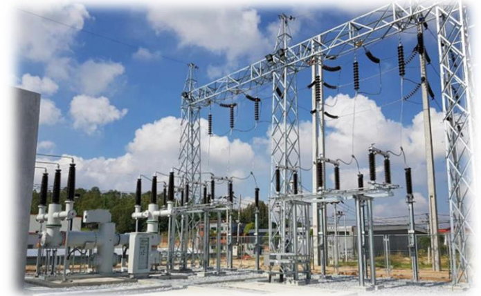
Power Substation Project
